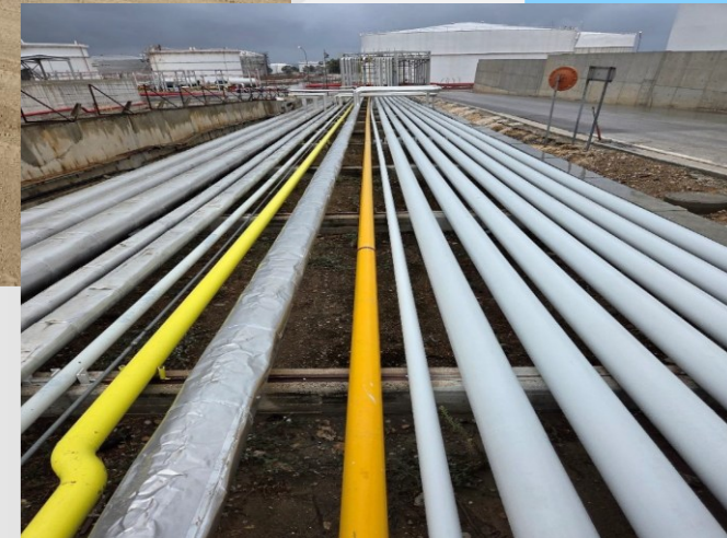
New Hydrogen Network Pipeline
